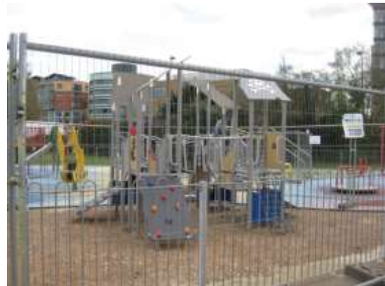
Fig.1(d). Barriers round new installations.
