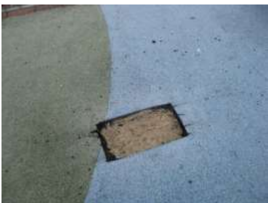
Fig.2. Small patch where flooring is missing.
