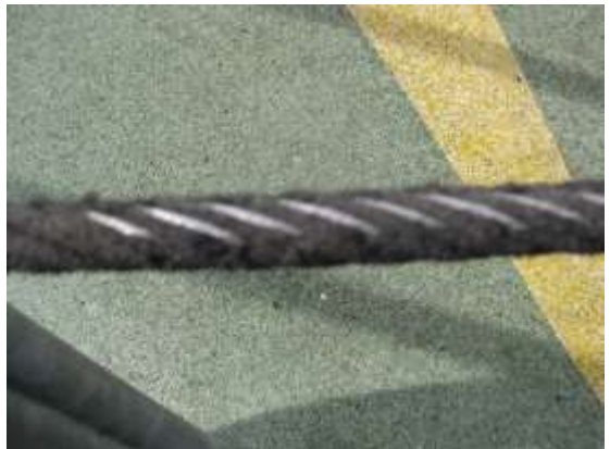
Fig.5(f). Metal rope exposed.
