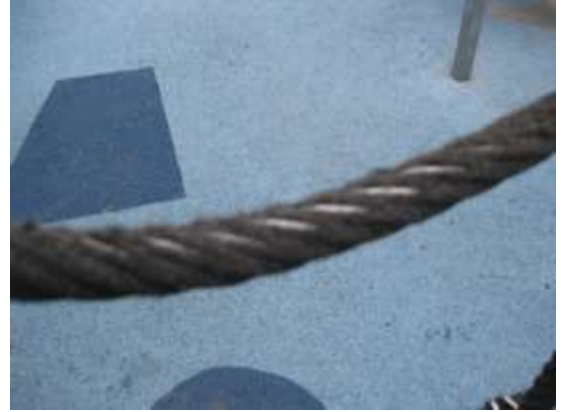
Fig.6(b). Metal rope exposed.
